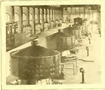
Generator room of the Niagara Falls Power Company.
